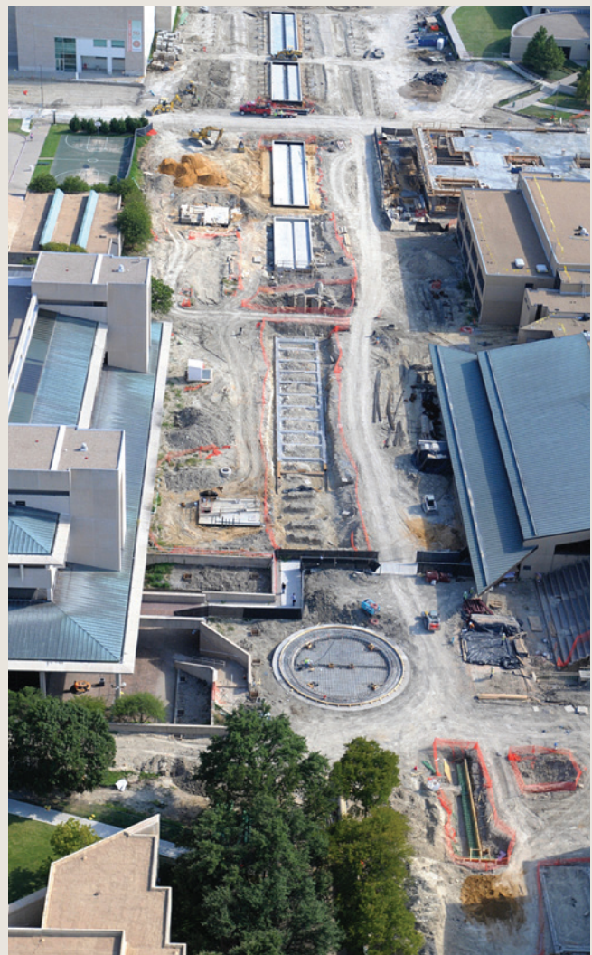
Ten months after the formal groundbreaking in November 2008, the Campus Enhancement landscaping project dominated the central campus, looking south with McDermott Library on the left and the Student Union on the right.
