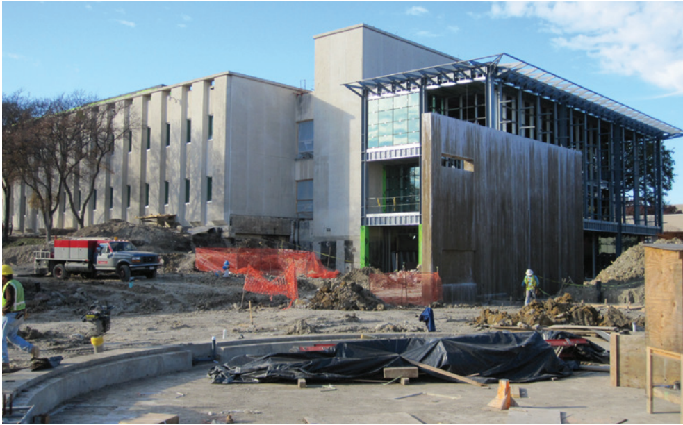
The multi-year renovation of Founders Building began in winter 2003. It required careful planning to accommodate the relocation of sensitive laboratory equipment and ongoing experiments.
